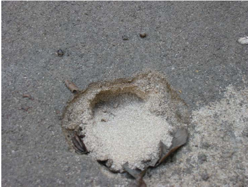
Figure 7 Formation of Clogging Crust on Filter Bed
